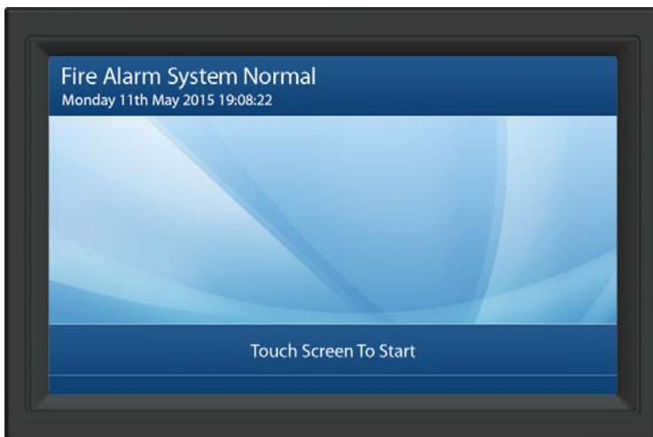
Figure 1-2 Normal-Standby-Condition of Touch-Panel-Display
