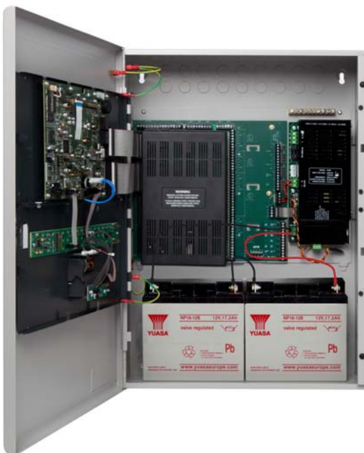
Figure 2-11 Connecting Standby-Batteries of the 5.25 Amp Power Supply
