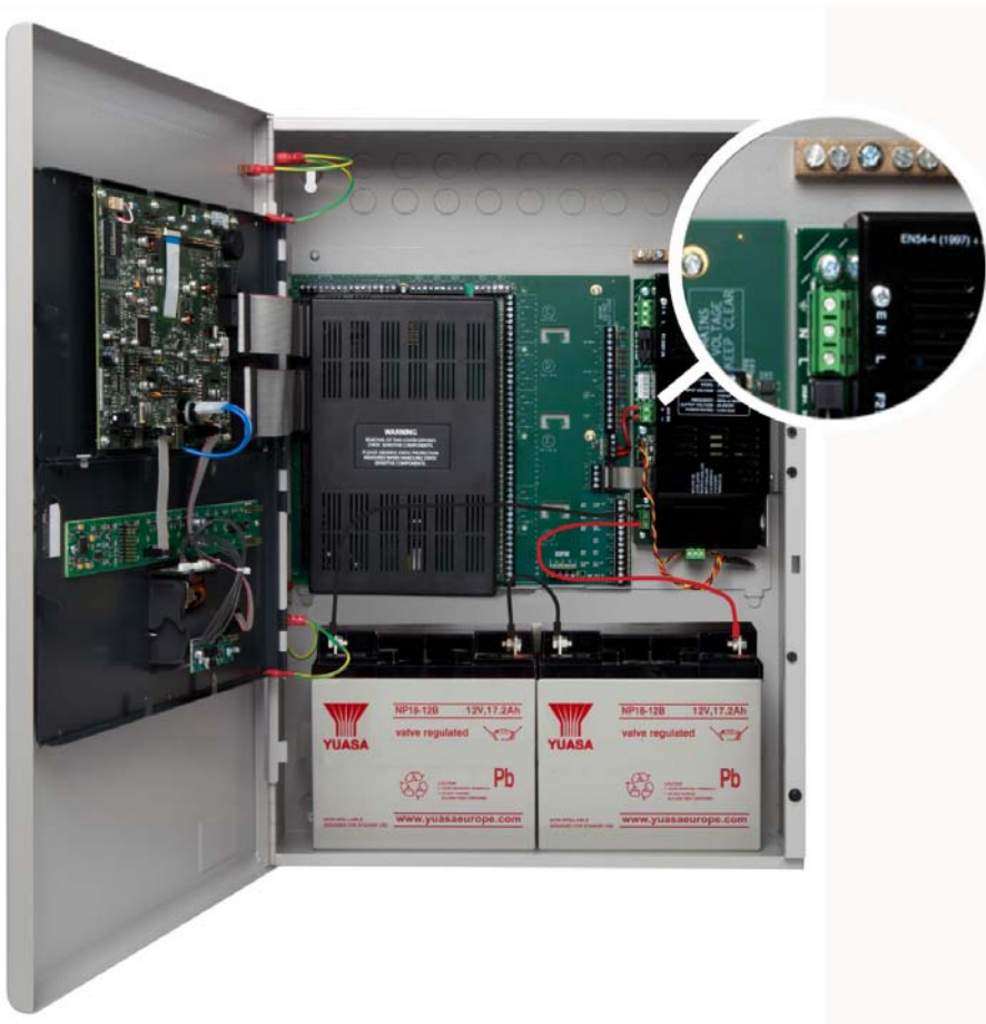
Figure 2-15 AC Power Connections of the 5.25 Amp Power Supply
