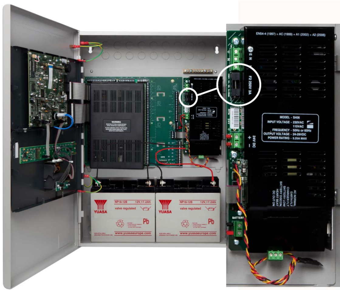
Figure 3-2 3 Amp Power Supply Fuse
