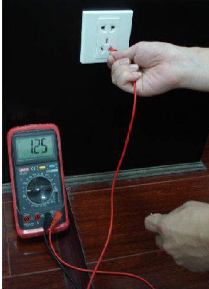
Appendix Figure 7-6 Check live cable connection
